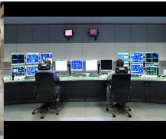
FLSmidth Control Room
